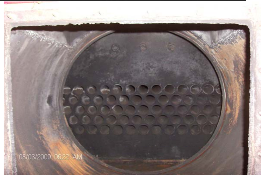
Before cleaning in August with Fitch running since late June Even then it was showing signs of self cleaning.
