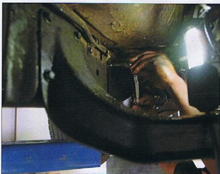
Holes were then drilled into the frame and tapped to create a secure mounting position for the Fitch unit.
