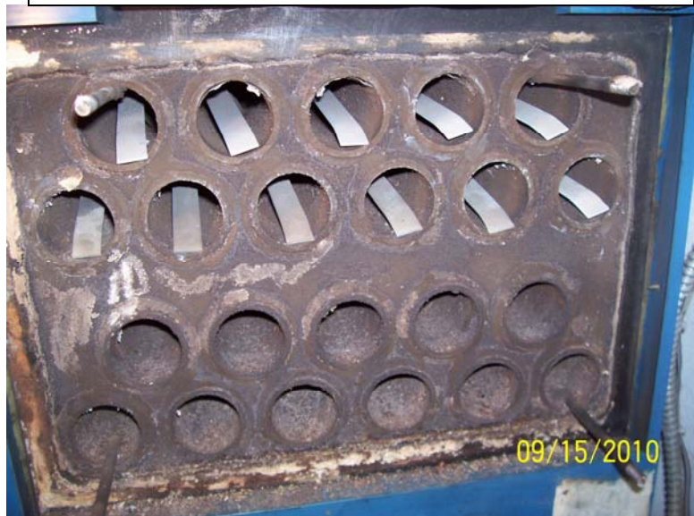
Photo #2 September 15, 2010 – 2 nd Re-inspection After Fitch Fuel Catalyst installation Residual carbon is virtually gone
